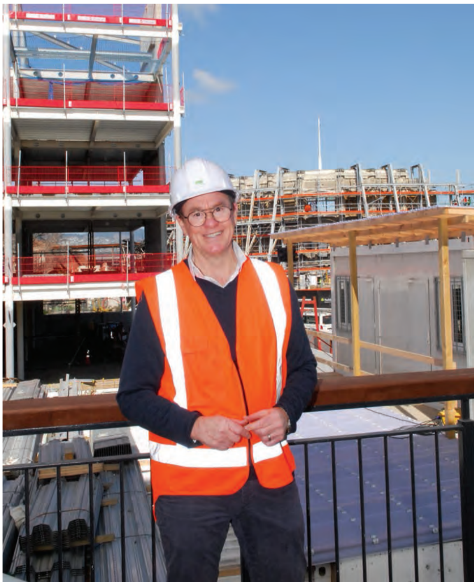
Work in progress at the Innovation Precinct: Visible behind CCDU’s Don Miskell (at Dux Central) is the Vodafone building (red scaffolding) and the McKenzie and Willis façade (in the background) where planned lanes and courtyards will create vibrant social spaces.
