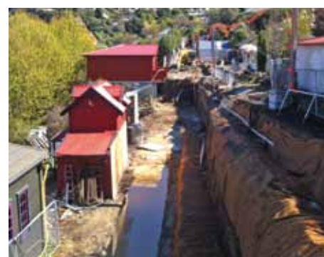
Cunningham Terrace, Lyttelton: the retaining wall is being rebuilt using ground anchors to increase its strength.
