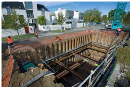
The Chester Street West Pump Station during construction, showing the sheet piling in place.
