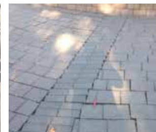
20 Lateral spread damage to paving.
