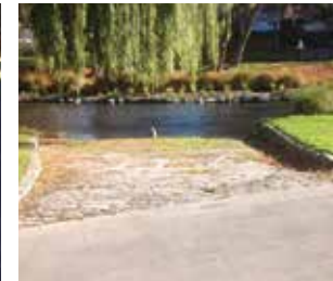
8 Damaged ramps and heritage walls.
