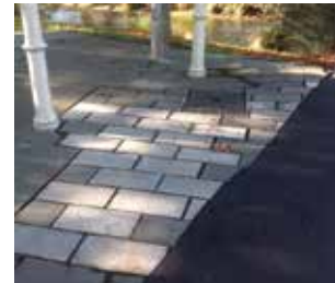
1 Uneven surfaces, broken pavers.
