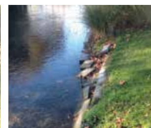
57 Damaged river walls.
